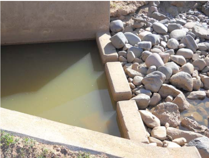
PHOTO NUMBER: 5 PHOTO DIRECTION: East DESCRIPTION: Stilling basin and wing walls. Appears free of cracks and spalls.
