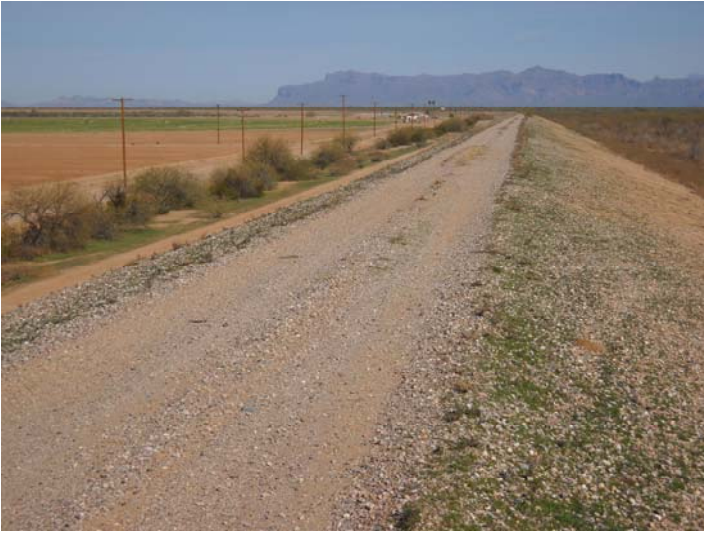
PHOTO NUMBER: 21 PHOTO DIRECTION: North DESCRIPTION: Crest of dam and upstream slope (west leg).
