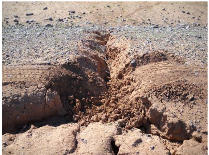
PHOTO NUMBER: 12 PHOTO DIRECTION: South DESCRIPTION: Transverse crack in crest.
