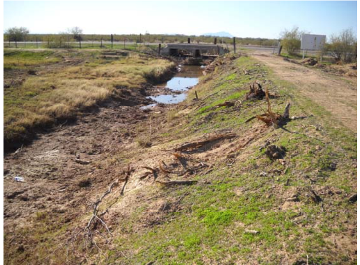
PHOTO NUMBER: 2 PHOTO DIRECTION: South DESCRIPTION: Outlet channel with access gate at right. Bridge is on Arizona Farms Road.
