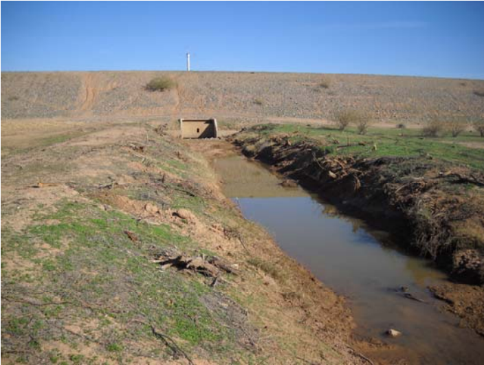
PHOTO NUMBER: 1 PHOTO DIRECTION: North DESCRIPTION: Outlet channel. ALERT gage can be seen on crest of dam. Recently cleared of brush.
