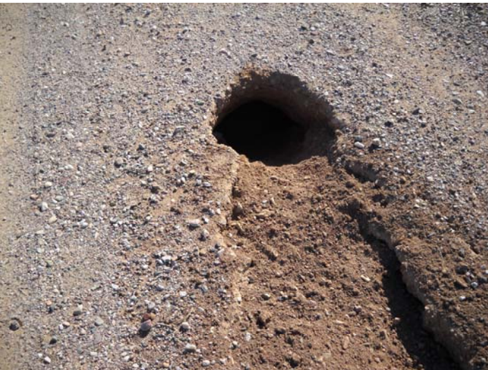
PHOTO NUMBER: 15 PHOTO DIRECTION: NA DESCRIPTION: Rodent burrow within crack.
