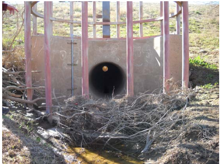
PHOTO NUMBER: 16 PHOTO DIRECTION: South DESCRIPTION: Inlet structure, conduit and trash rack.
