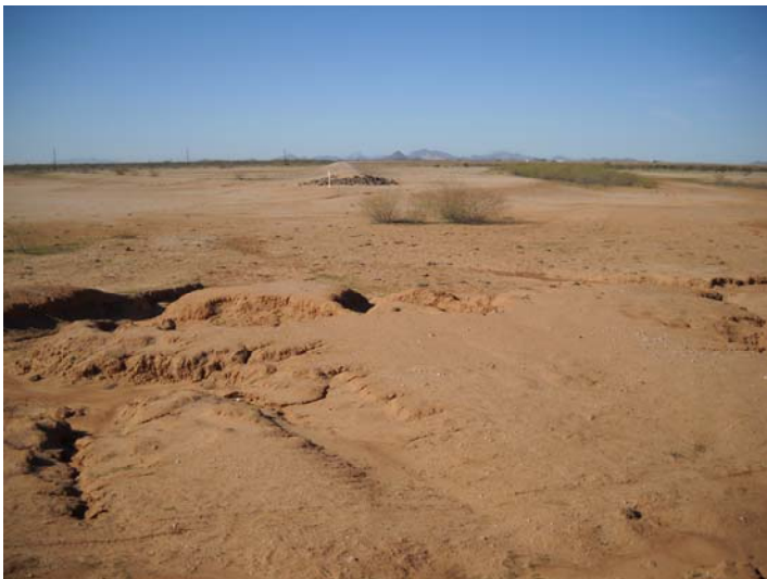
PHOTO NUMBER: 7 PHOTO DIRECTION: West DESCRIPTION: Looking across emergency spillway control section at left end of dam (riprap). In foreground is training dike.
