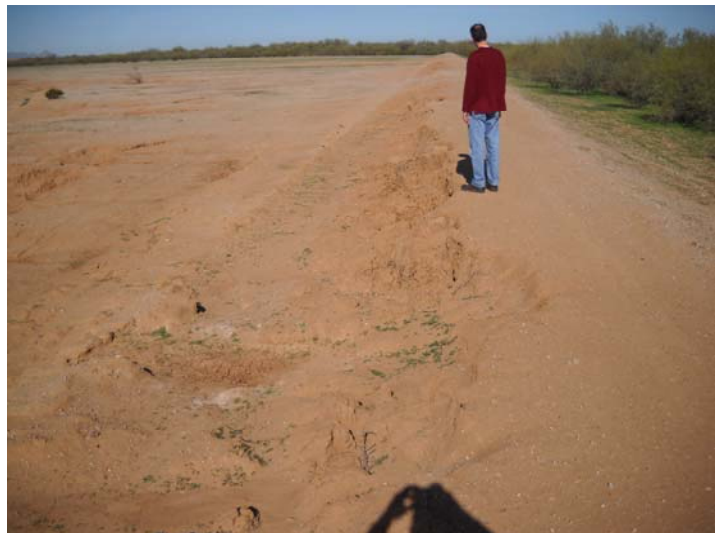
PHOTO NUMBER: 8 PHOTO DIRECTION: North DESCRIPTION: Emergency Spillway training dike shows signs of heavy local rain/surface flow as evidenced by erosion.
