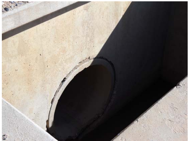
PHOTO NUMBER: 4 PHOTO DIRECTION: Northeast DESCRIPTION: RCP at outlet structure. Open and clear as shown in photo 16.
