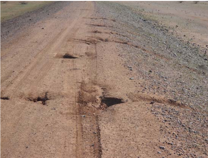
PHOTO NUMBER: 9 PHOTO DIRECTION: East DESCRIPTION: Crest of dam with transverse cracking and erosion.
