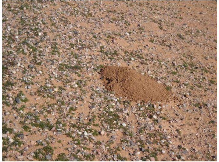
PHOTO NUMBER: 22 PHOTO DIRECTION: NA DESCRIPTION: Rodent burrow on upstream slope.
