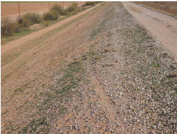
PHOTO NUMBER: 23 PHOTO DIRECTION: North DESCRIPTION: Downstream slope west leg of dam.
