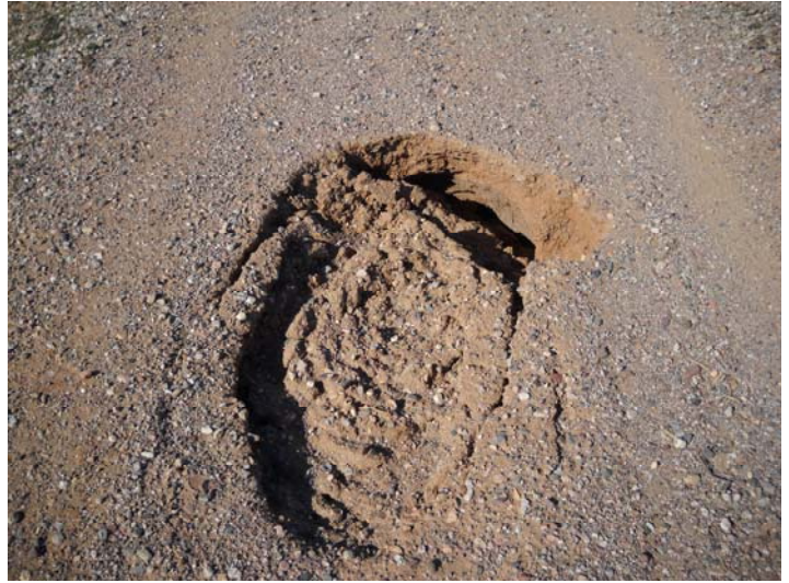
PHOTO NUMBER: 14 PHOTO DIRECTION: NA DESCRIPTION: A developing sinkhole on crest.
